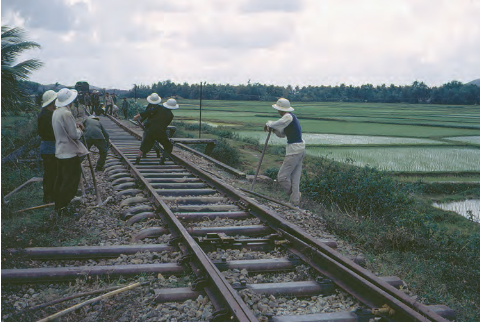
South Vietnamese railway workers repair tracks between Qui Nhon and Phu Cat.
